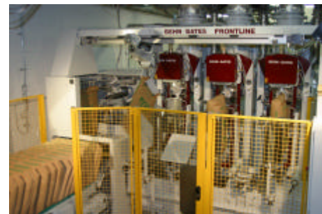
Automatic filling plant with FRONTLINE valve bag applicator, 3 pneumatic packers and ultrasonic valve bag sealing stations for sugar
